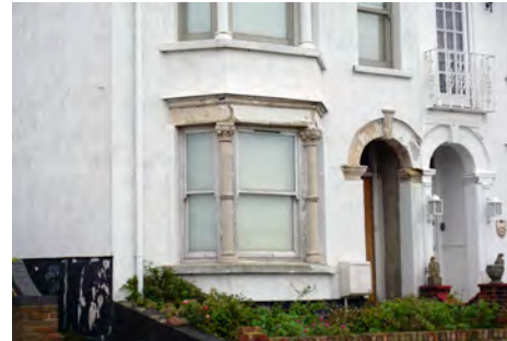
Examples of Poor Decorative Condition
