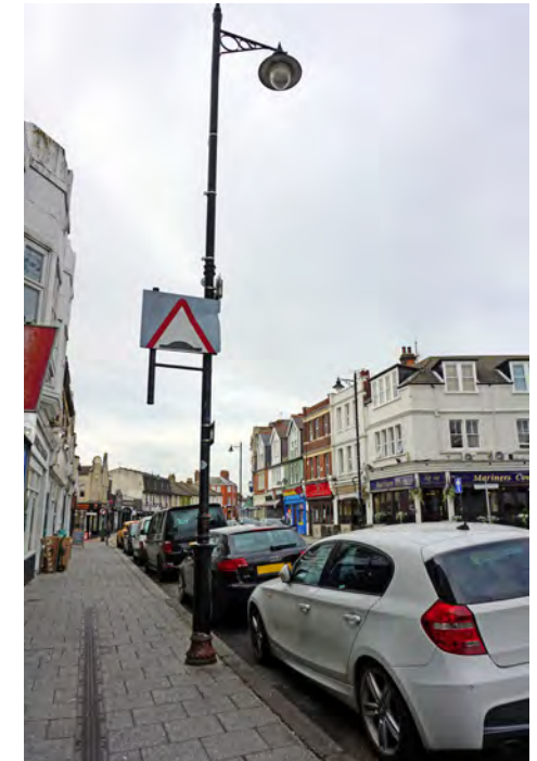
Good traditional lamppost on Broadway but with a damaged and intrusive sign attached
