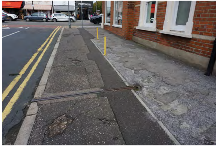
Poor surfacing and dominant yellow lines
