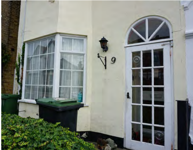
Infilling of porch with door that has an overemphasis on glazing and uPVC windows with top hung casements and the loss of stone mullions to the bay
