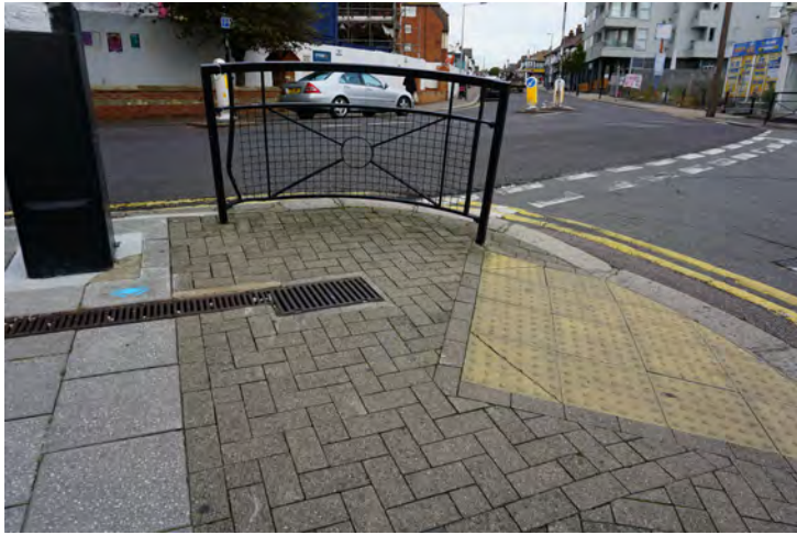
Damaged railings on Broadway
